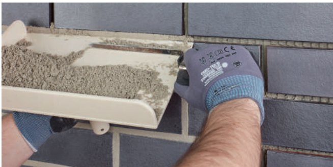
Traditional joints to be pointed
